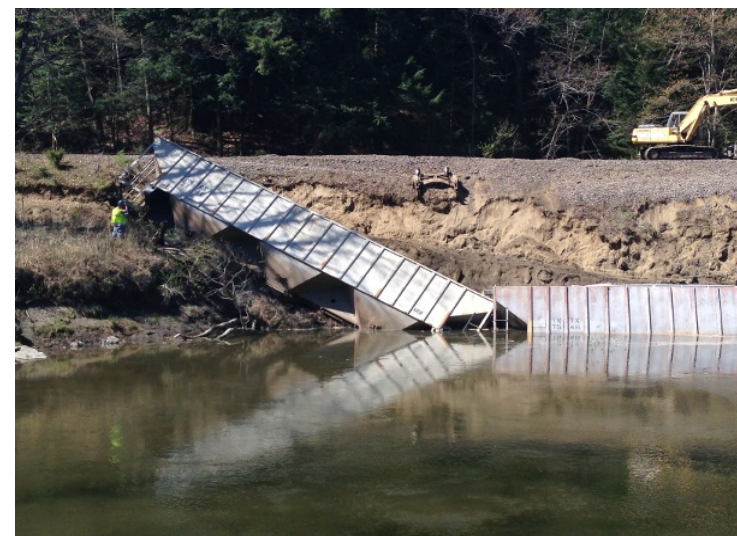
Three railroad cars carrying corn fell into the Passumpsic River in East Barnet in May, 2013 due to bank erosion.
